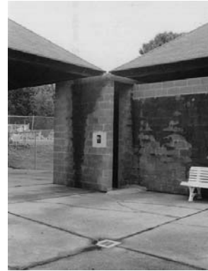
Typical water damage, Trenton Bath House, Trenton, NJ (photo: Susan Solomon)
